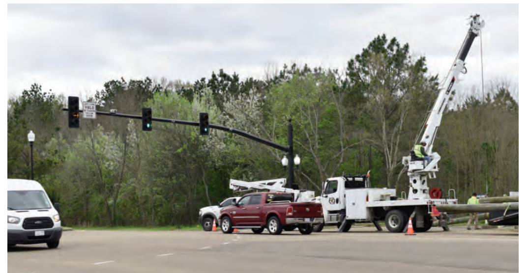
Crews finalize new traffic lights on Highland Colony Parkway that will be tested for 30 days.
