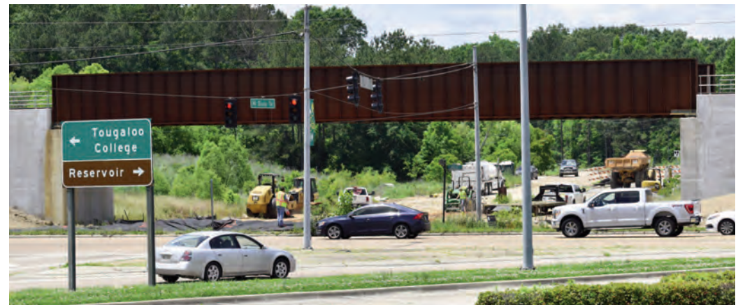
An $8 million realignment of the Canadian National Railroad is nearing completion. The project began in 2016.
