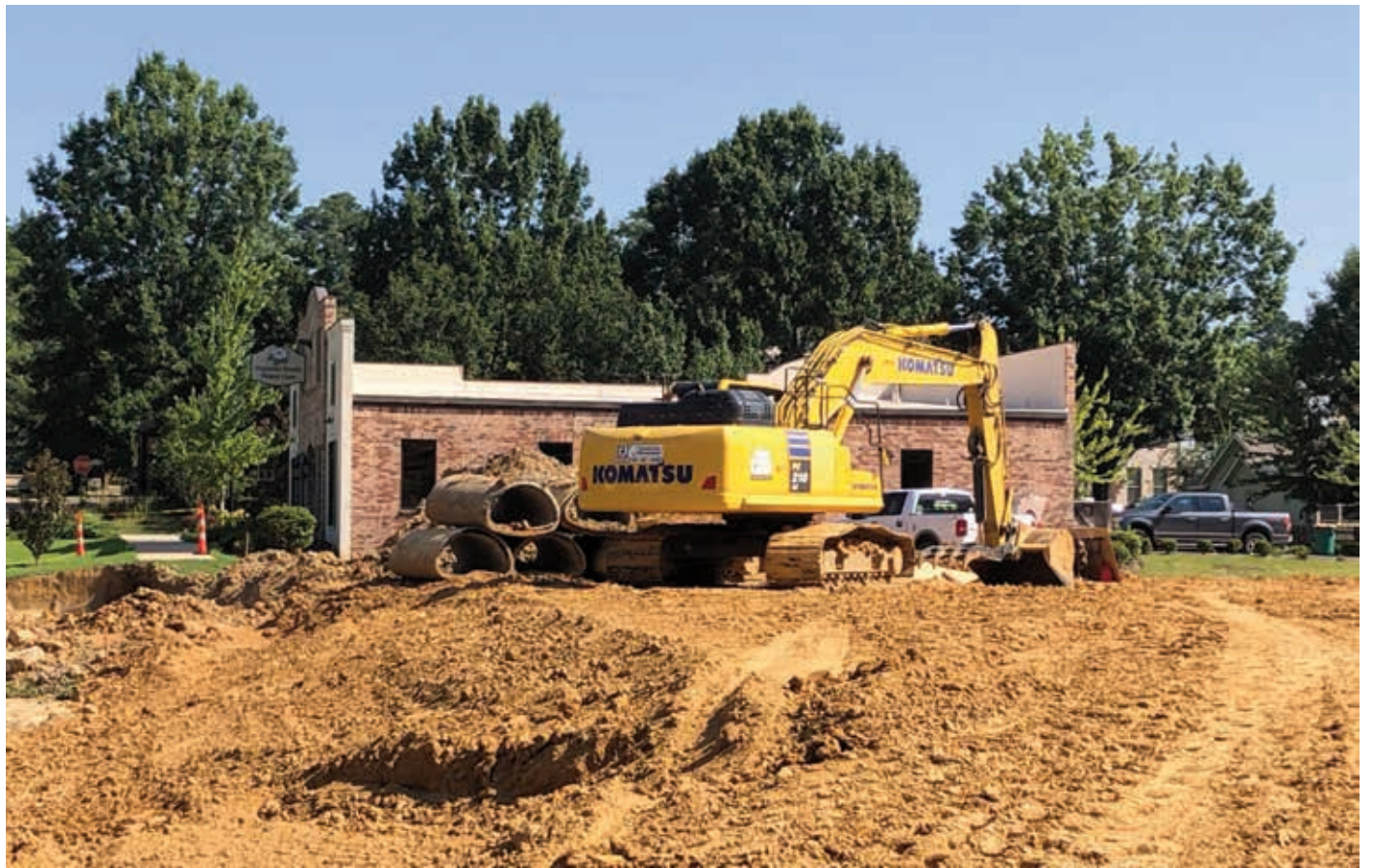
Dirt work is underway at a new shopping center in Ridgeland's Olde Towne.
