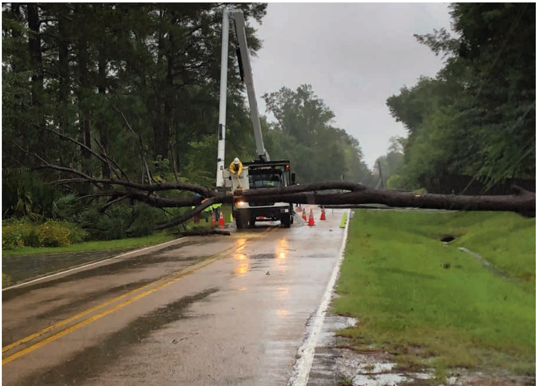
A lineman hacks his way through a tree that fell on North Old Canton Road in Madison Monday, knocking out power to approximately 1,200 houses.
