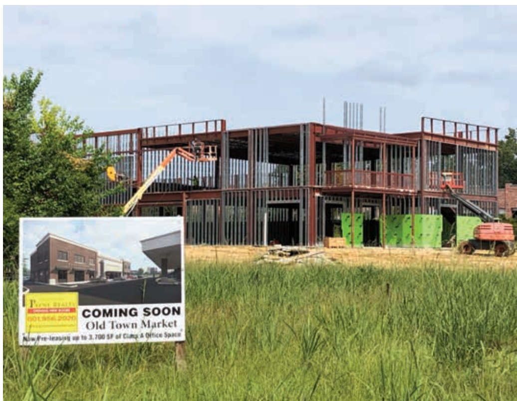
Construction crews work on the site of the new Old Town Market in Ridgeland.
