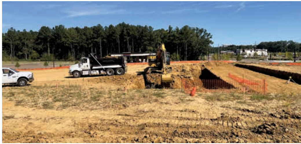
Dirt work has begun at the site of the new Highland Colony Chick-fil-A.
